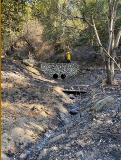
Road crossing near Millard Campground have potential for culverts to plug
