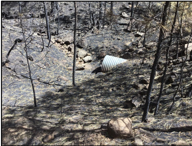
Figure 5. Burned area above culvert where increased erosion and sedimentation can plug culverts leading to a road being overtopped by flood waters.
