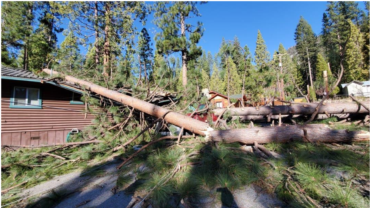
Building in Wawona damaged by trees that fell during Mono winds on January 19, 2021 (Photo: National Park Service)
