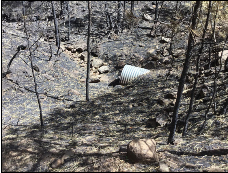
Figure 5. Burned area above culvert where increased erosion and sedimentation can plug culverts leading to a road being overtopped by flood waters.
