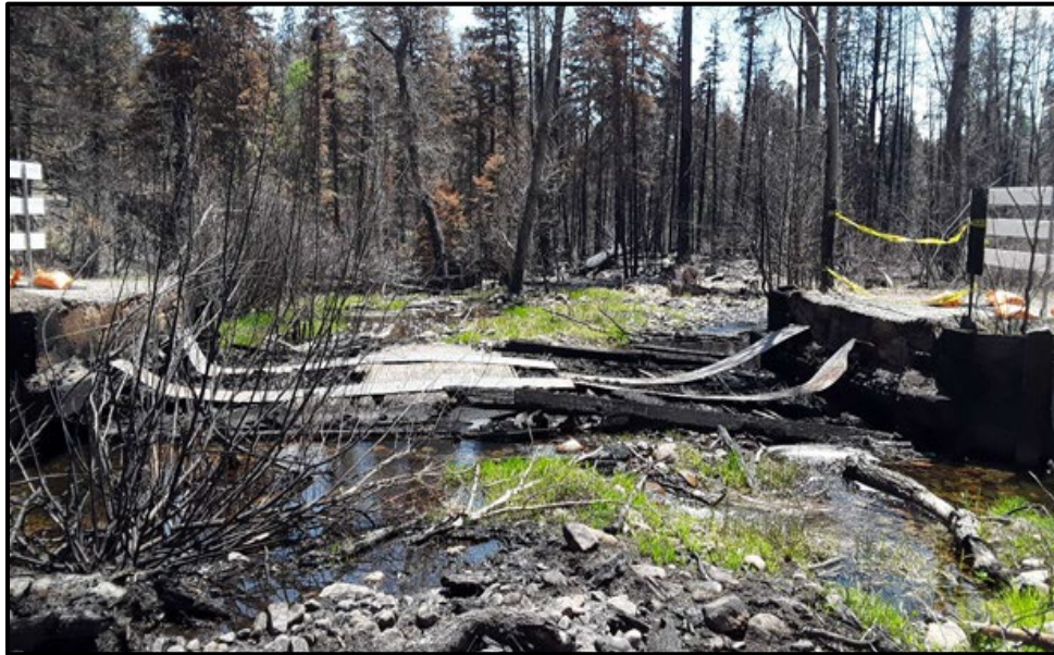
Figure 6. Burned infrastructure that may mobilize during a storm.
