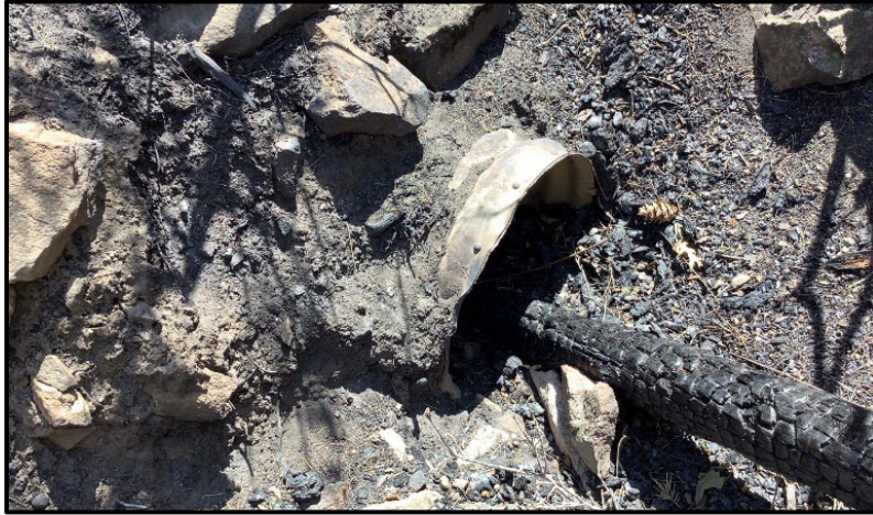
Figure 5. Plugged culverts can lead to a road being overtopped by flood waters.
